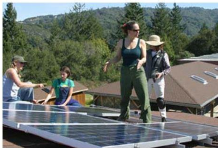
Solar Energy International sponsored a workshop at Walden West Outdoor School.. A group of 23 women, including (from left) Michelle Large, Nicole Clock, Angie Stuart and Kate Lathan, installed solar panels at the school.
